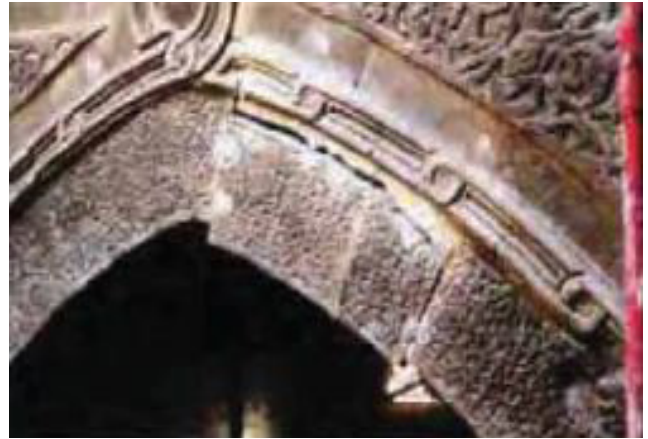
Seismic damage to decorative arches
