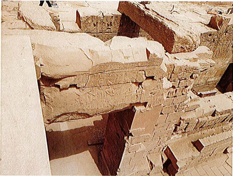
Side elevations and top view of cracked architrave
