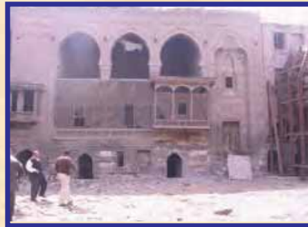
Typical damaged facade
