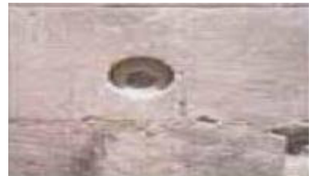
One of the four arches of the court being scaffolded prior to drilling and anchoring.
