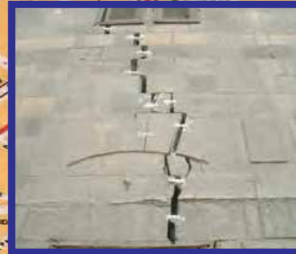
Typical damage caused to exterior walls
