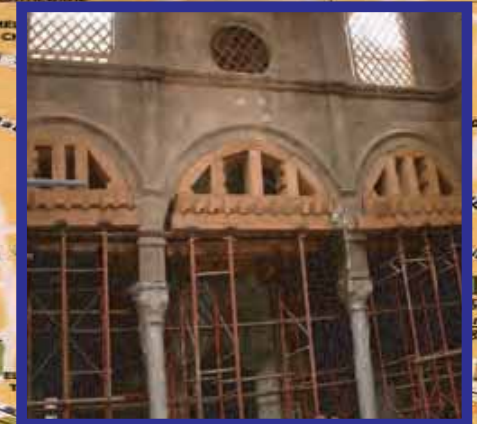
Buckling and movement of columns
