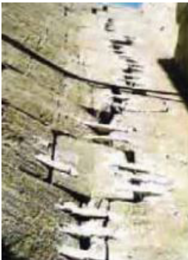
Vertical shear crack
