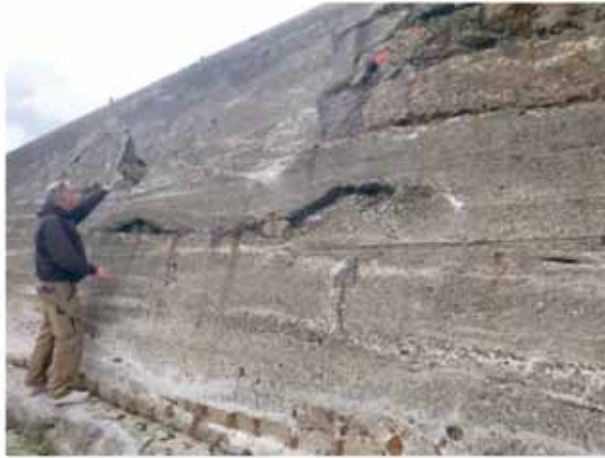
Figure 6. Poor surface of WWII wall with inclusions
