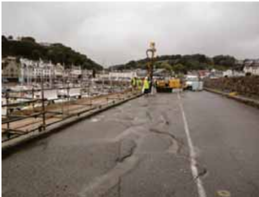
North Pier - cracks at deck level
