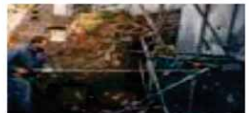
The process of diamond drilling (below). With the subsequent core samples produced, (left).
