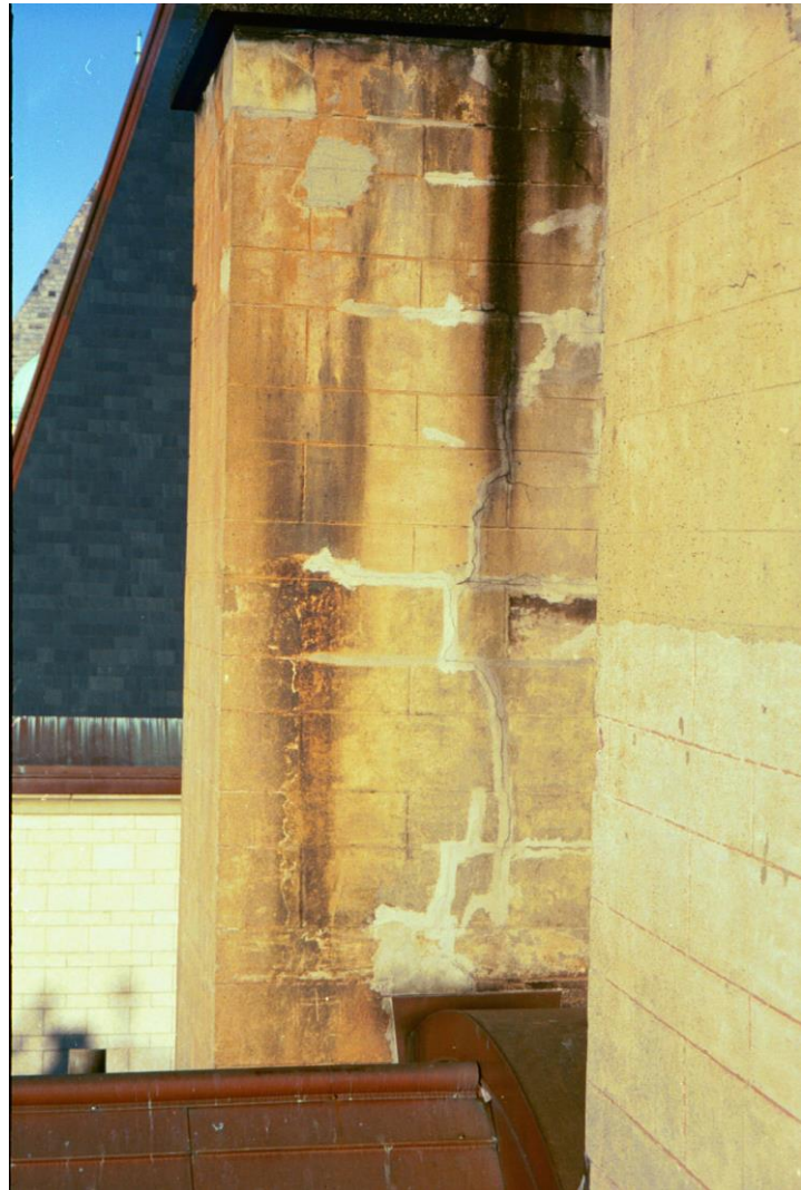
Failure due to hard mortar repointing
