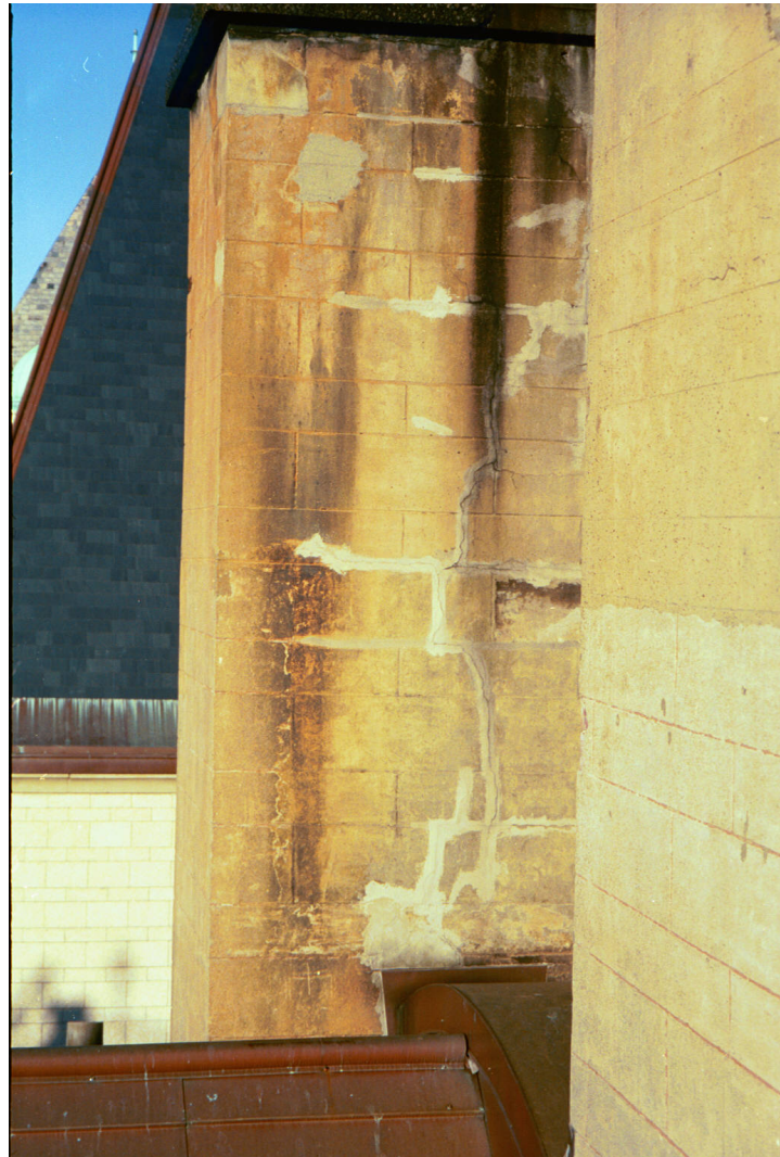
Failure due to hard mortar repointing
