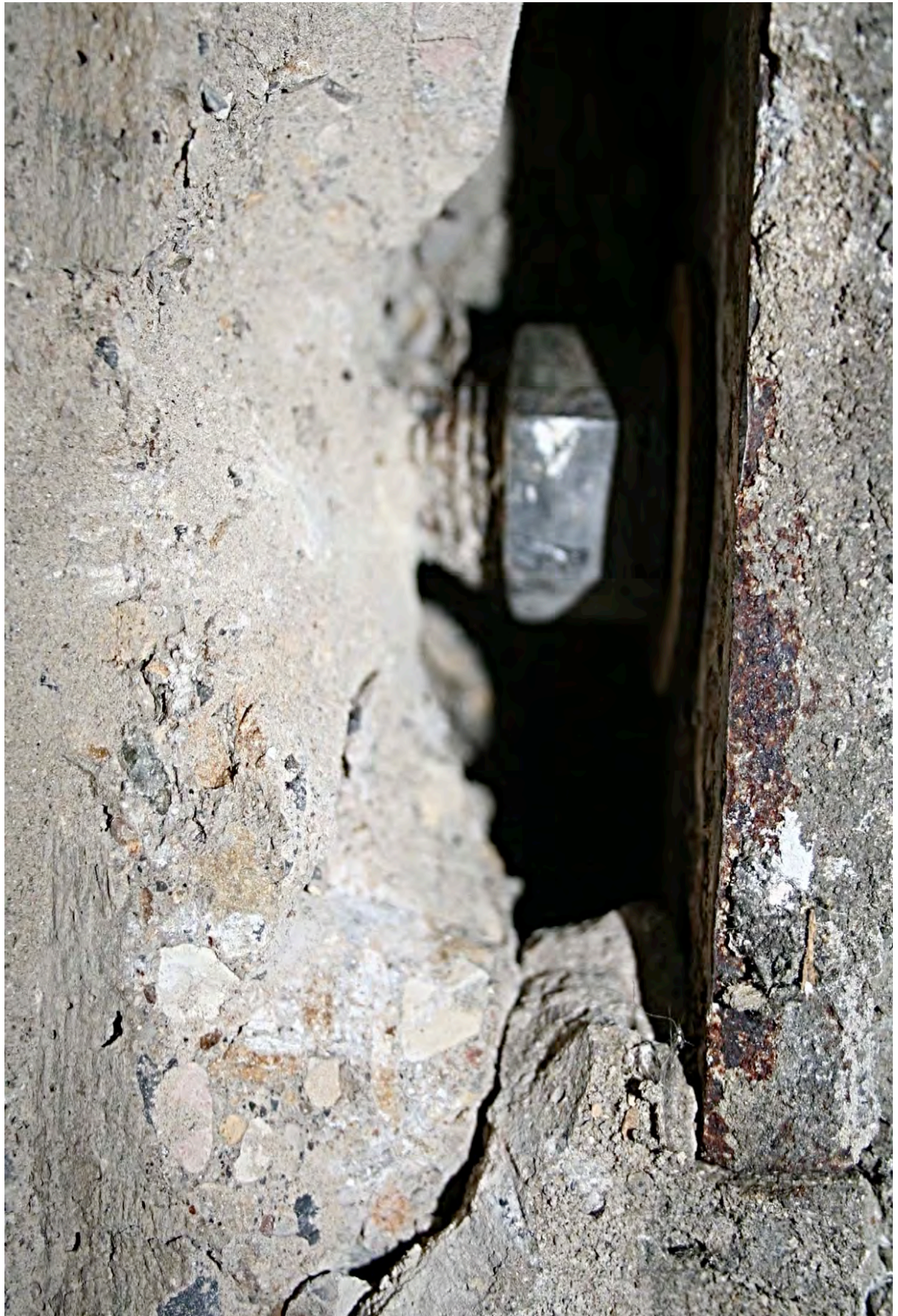
Original levelling bolt when the units were positioned. Photograph 6
