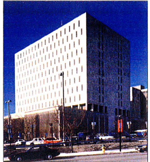
Limestone cladding of Essex County New Courts Building and Jail was one accident away from catastrophic failure. More than 20,000 Cintec anchors now prevent masonry's collapse.
