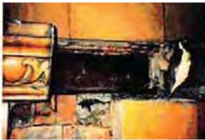
Example of steel beam corrosion causing failure of the decorative terra cotta facade.
