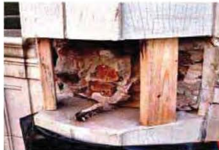
Corroded restraint fixing.
