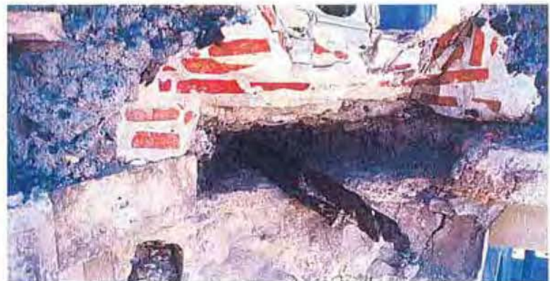
Once the cornice had been partially disassembled, the materials and techniques used in its construction could be easily identified. Note the clinker concrete, or "cindercrete," between the terra-cotta blocks and the brick backup material, and the severe deterioration of the steel supports. CSI recommended that all new steelwork be AISI Type 316 stainless steel, a non-corroding type, which is essential in this chloride-rich maritime environment.
