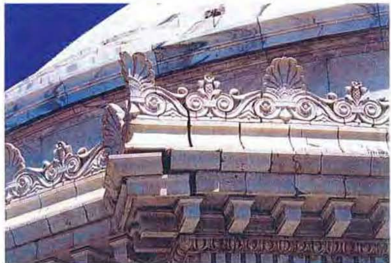
The poor condition of the terra-cotta cornice is evident in this view. The separation of the terra-cotta units is due to not only the failure of the anchoring system, but also the expansion of the corroded material.
