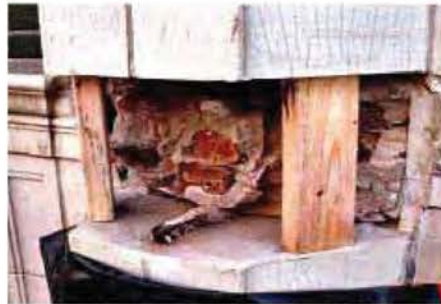
Corroded restraint fixing.
