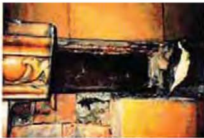
Example of steel beam corrosion causing failure of the decorative terra cotta facade.
