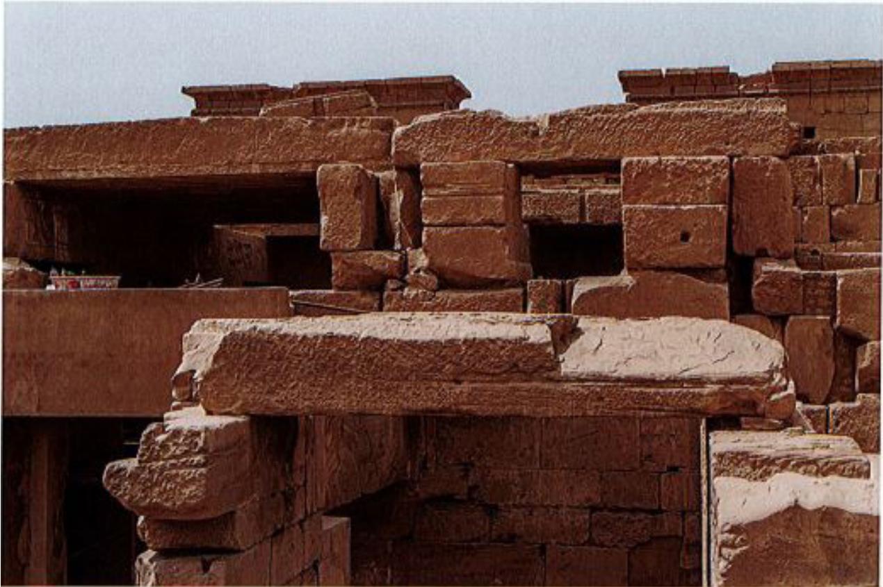
South Architrave, the one face had almost completely delaminated.
