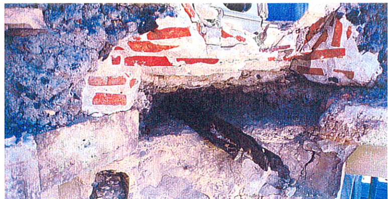
Once the cornice had been partially disassembled, the materials and techniques used in its construction could be easily identified. Note the clinker concrete, or "cindercrete," between the terra-cotta blocks and the brick backup material, and the severe deterioration of the steel supports. CSI recommended that all new steelwork be AISI Type 516 stainless steel, a non-corroding type, which is essential in this chloride-rich maritime environment.
