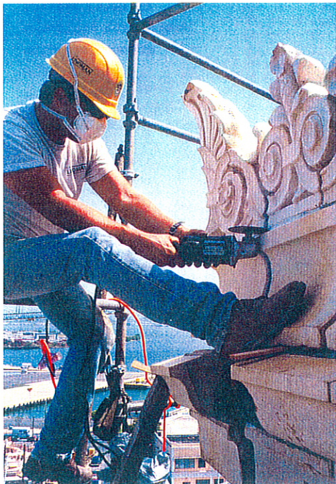
A worker is seen here cutting the mortar joints between the terra-cotta blocks in preparation for the disassembly of the cornice.
