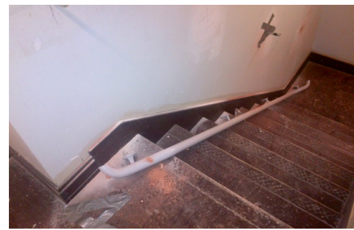
Two of the four anchors installed in the wall, note the exposed thread for attaching the handrail.
