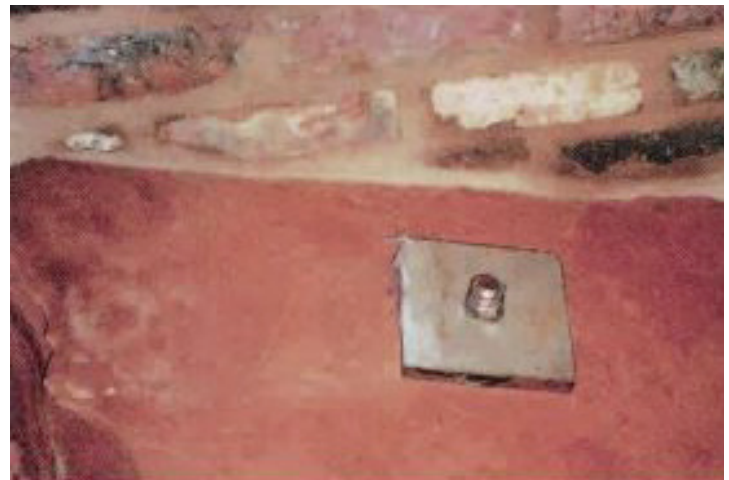
Roof bolt support to ballroom ceiling.
