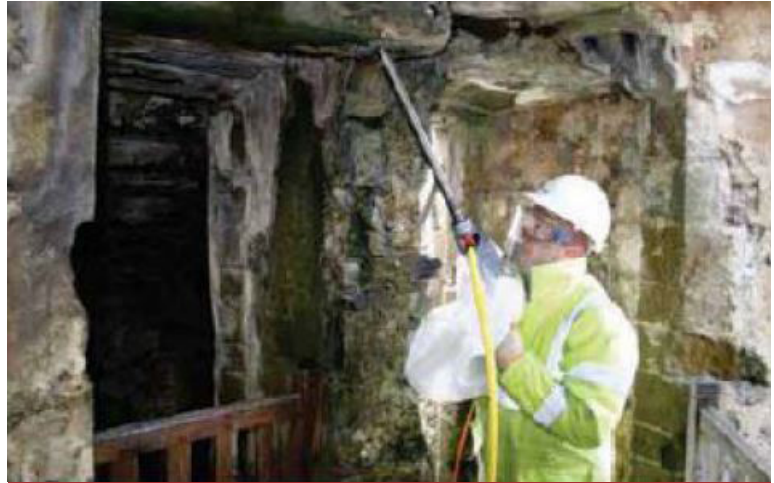
Diamond drilling to install anchors to secure a lintel over the doorway to the prison tower at Harlech.
