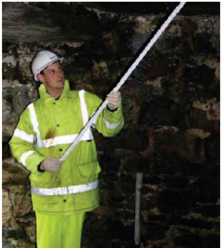
Installing anchor into diamond drilled hole to secure stones forming the floor/ceiling in the kitchen tower at Harlech.
