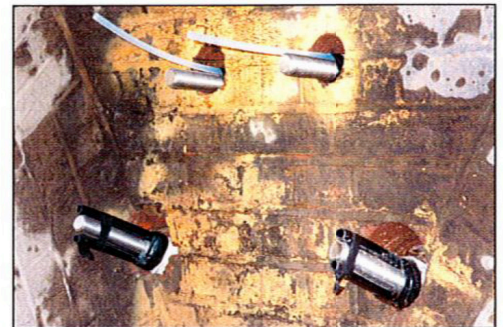
Shear anchors shown at the top and tension anchors at the bottom
