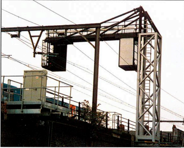
Cantilever Signal System
