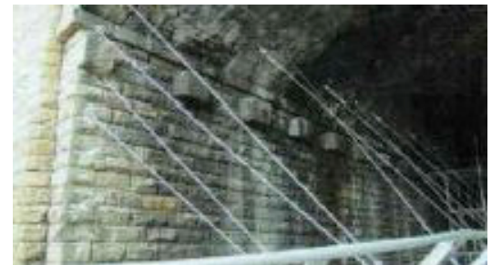
View of the supporting cables under the arch after lifting bridge from supporting scaffold.
