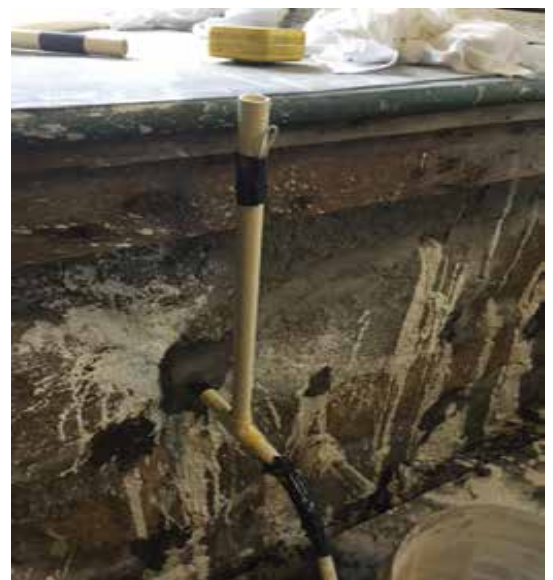
Fig. 10: In-line injection piezometer
