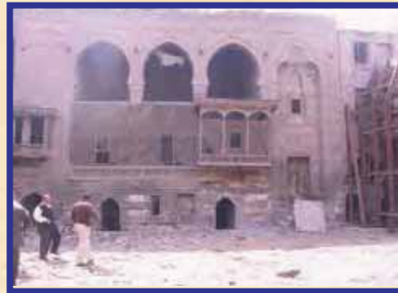
Typical damaged facade
