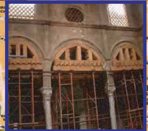
Buckling and movement of columns
