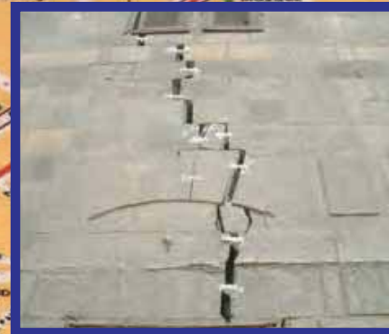
Typical damage caused to exterior walls
