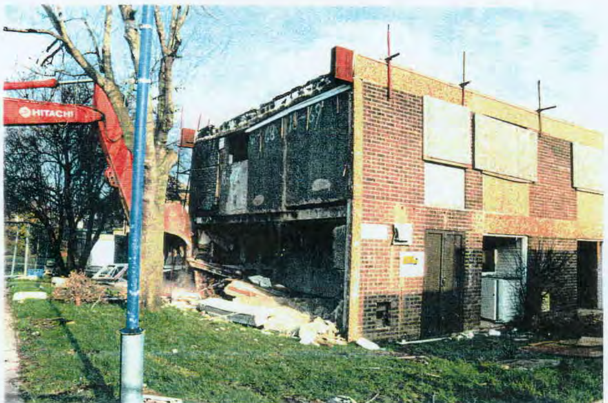
A5 The last remnants of the supports are removed and the first floor starts to fail slowly under the weight of the panels above.
