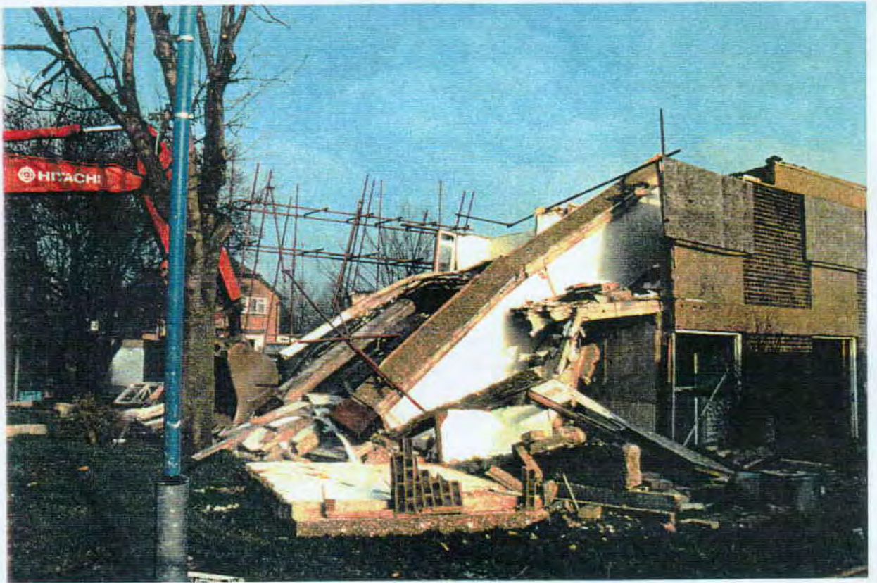
A35 Final condition of collapsed structure. Note most of the debris lies within the original dimensions of the building.
