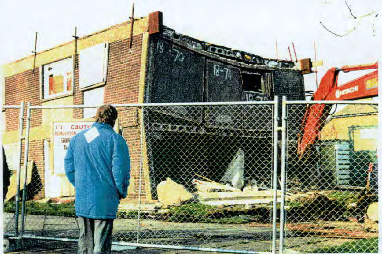
B6 The first floor is failing rapidly as the excavator bucket attempts to remove the remaining supports and the side walls have commenced buckling at first floor level.
