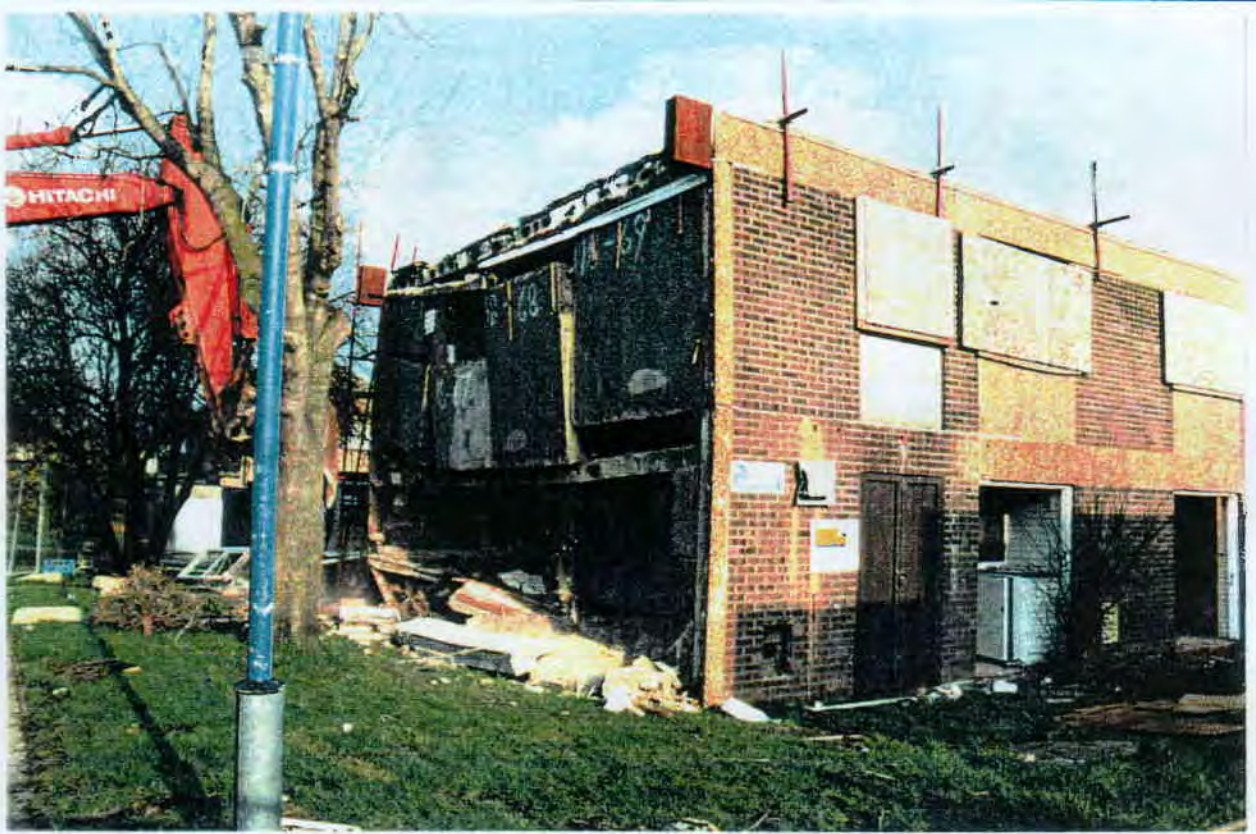
A8 The first floor continues to fail as a unit leaving behind the roof which is unsupported but still intact. The side walls start to buckle out at first floor level under rotational forces induced by the first floor wall panels.
