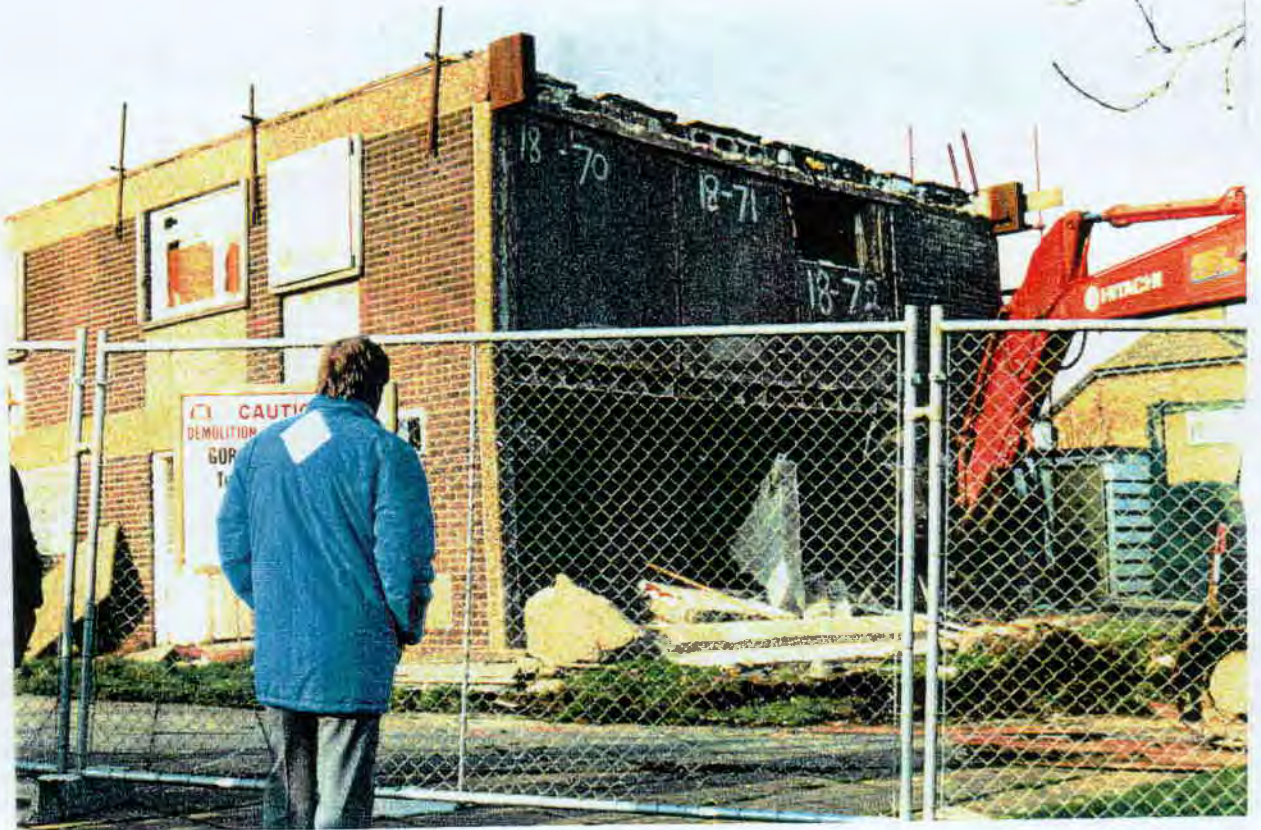
B5 This shows a stage where the support wall is being removed. It can be seen that the first floor has slipped down at the side nearest the camera and the end first floor wall panels and the side walls have started to rotate.
