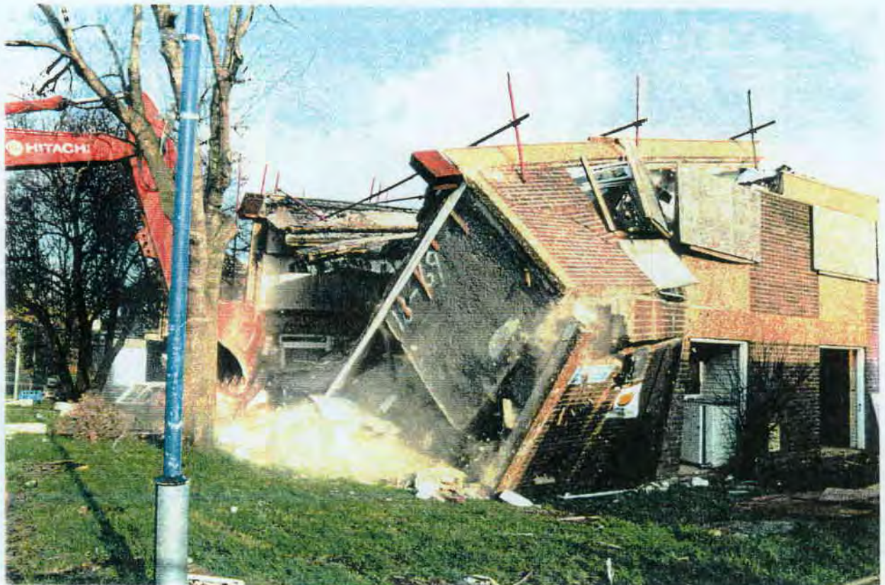
A14 Collapse of the complete end of the structure. Note the upper storey side walls being pulled inwards and roof now in free fall but still continuous.
