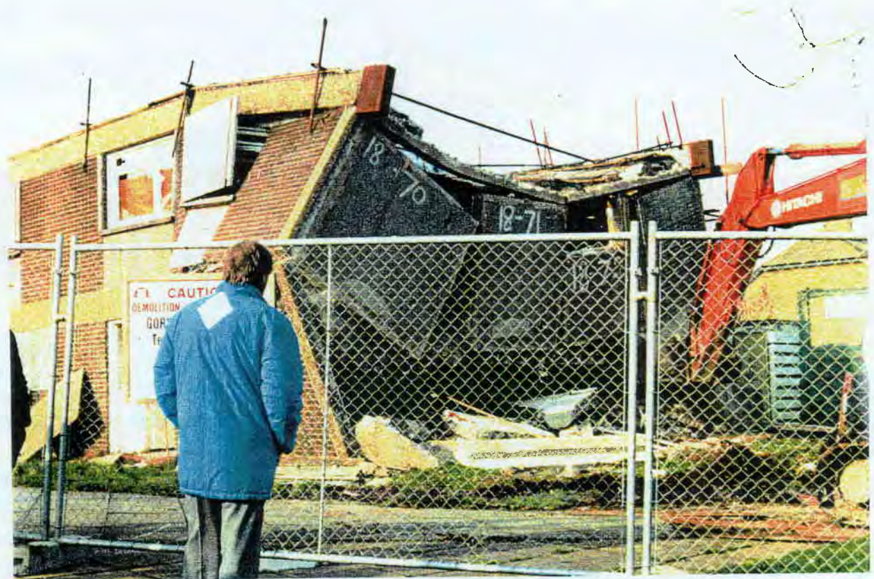
B8 The roof continues to follow the first floor in free fall.
