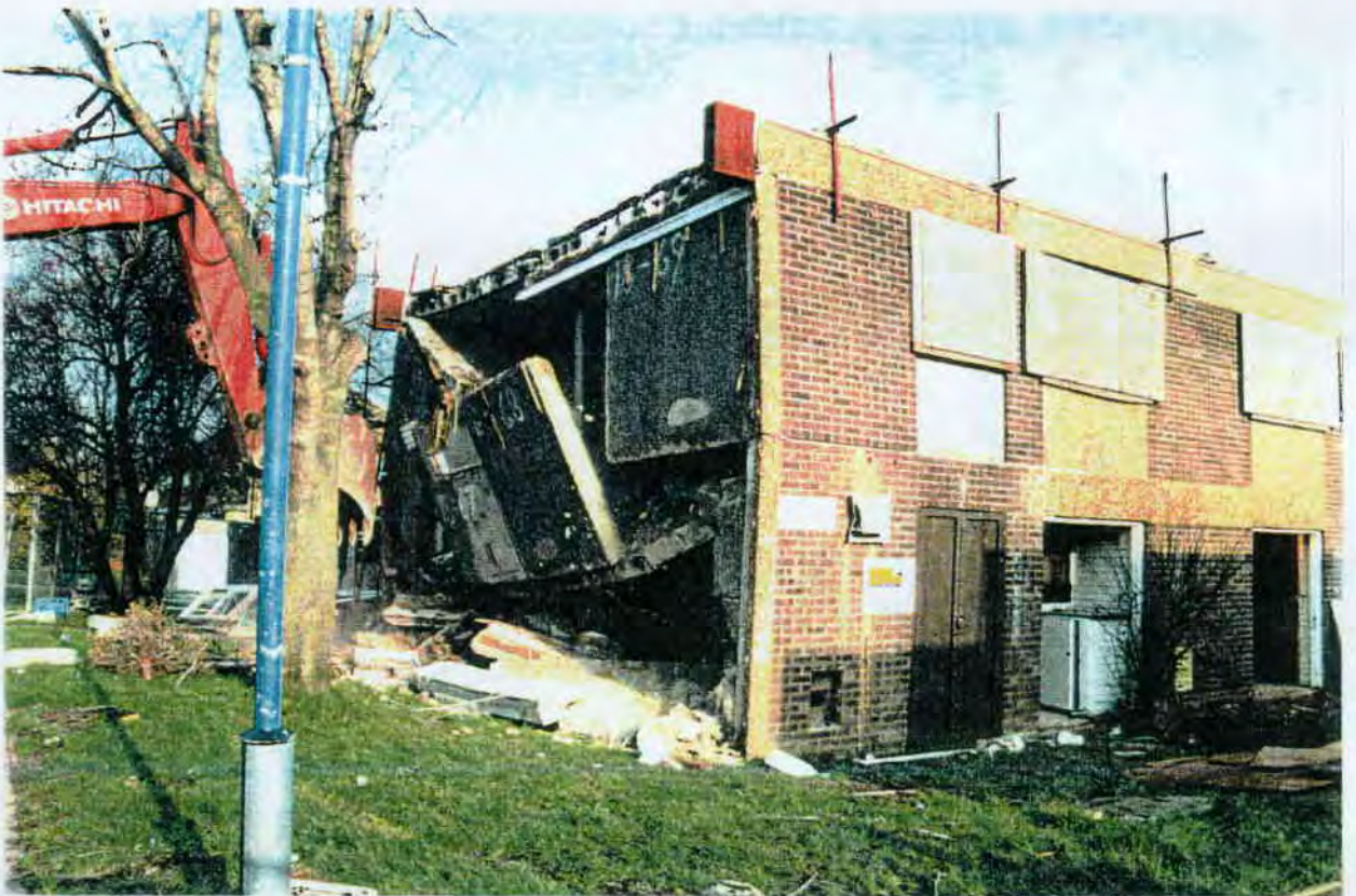
A10 The first floor collapse is complete, the side walls are now buckling badly but the unsupported roof remains in place and intact.
