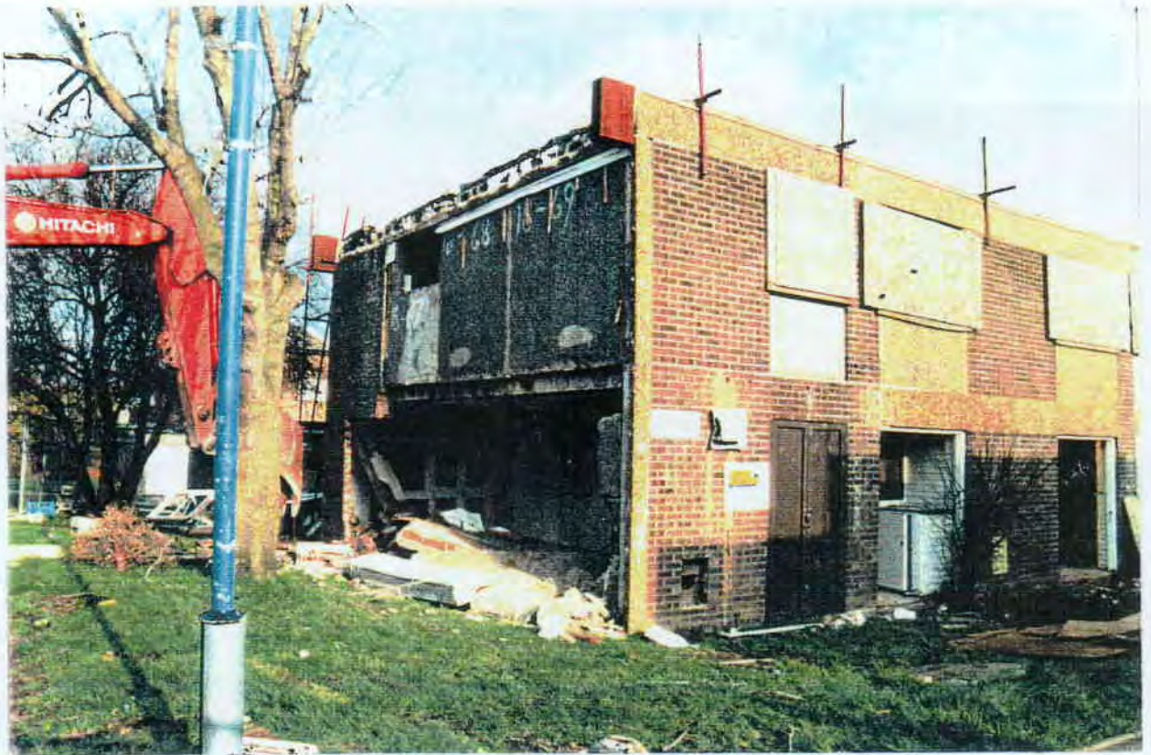
A4 Shows the stage where virtually all the load bearing support has been removed from the end of the structure. At this point there is no significant disruption to the structure and the first floor planks have just started to deflect under the load.
