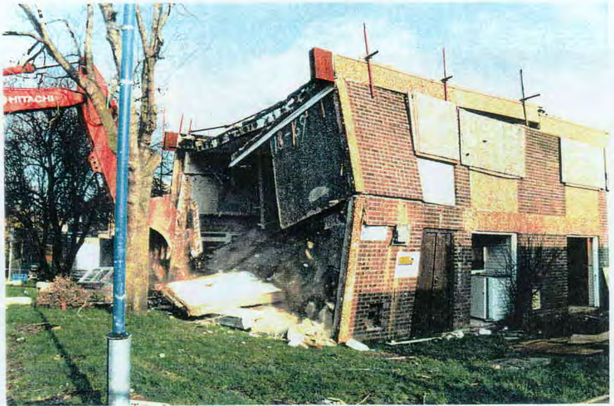
A12 There is complete loss of stability of the side walls due to rotation at first floor level forcing down the roof structure as a unit.
