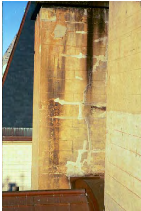
Failure due to hard mortar repointing.)
