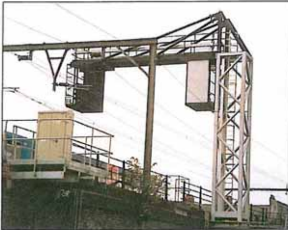
Cantilever Signal System
