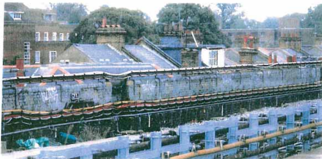
Figure 1 Parapet wall with bolted on utilities
