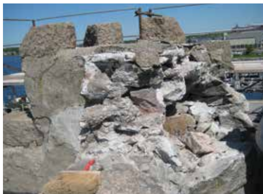
Fig. 2: Internal turret condition
