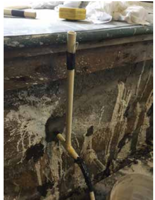
Fig. 10: In-line injection piezometer
