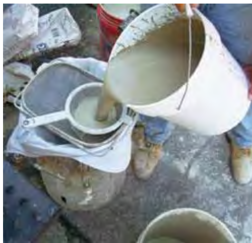
The masonry grout is strained to remove lumps before it is fed into the fabric sleeve.
