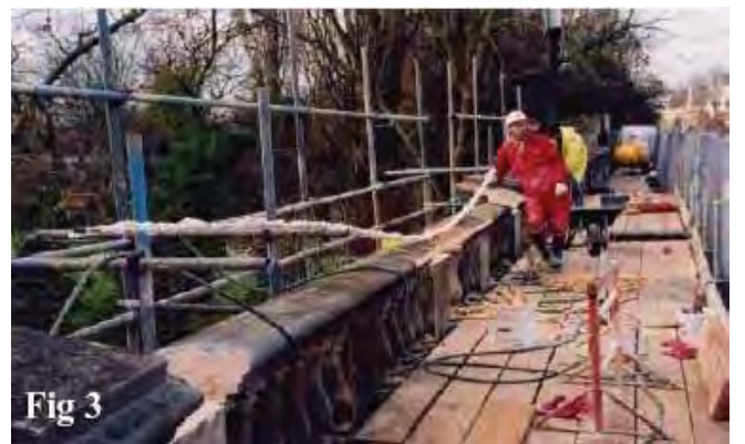
Figure 2 shows the holes drilled horizontally through the parapet. Figure 3 shows a horizontal Cintec anchor prior to installation
