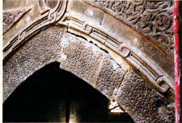
Seismic damage to decorative arches
