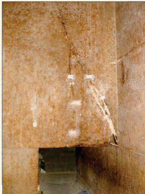
Front elevation of cracked beam
