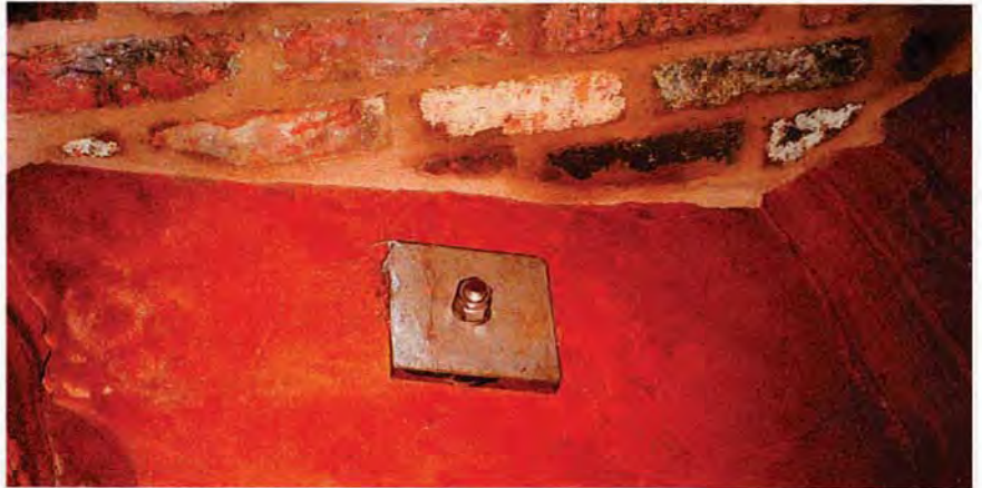
Roof bolt support to ballroom ceiling.
