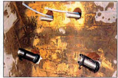
Shear anchors shown at the top and tension anchors at the bottom
