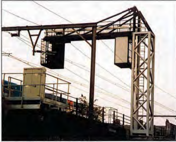
Cantilever Signal System
