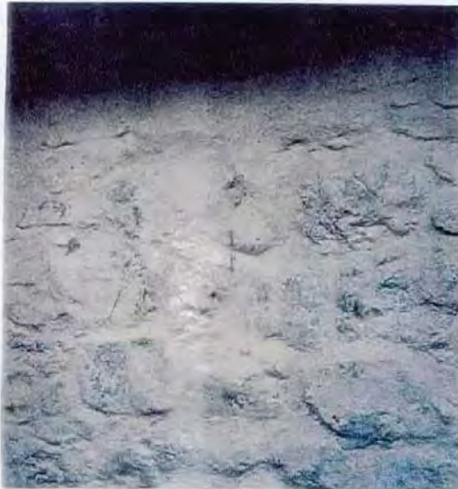
(g) The finished wall after installation of anchor and before white washing.
