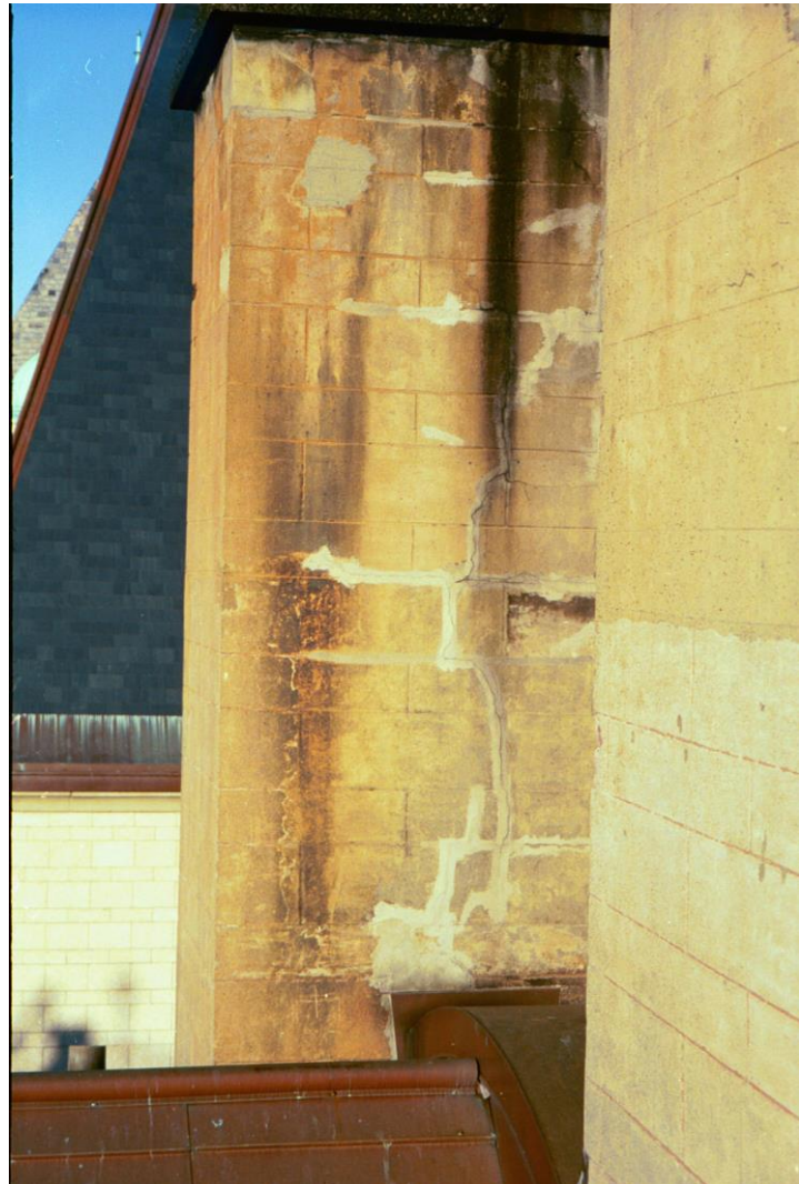
Failure due to hard mortar repointing
