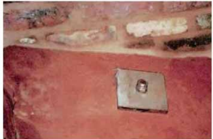
Roof bolt support to ballroom ceiling.
