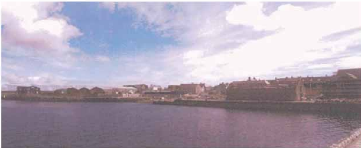
Panorama of Hay's Dock with the Heritage Centre under construction in the background (right), the restoration of the old sail house on the quay (centre right) and Cintec stabilisation work (end of the quay left of sail house).
