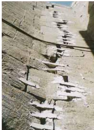
Vertical shear crack
