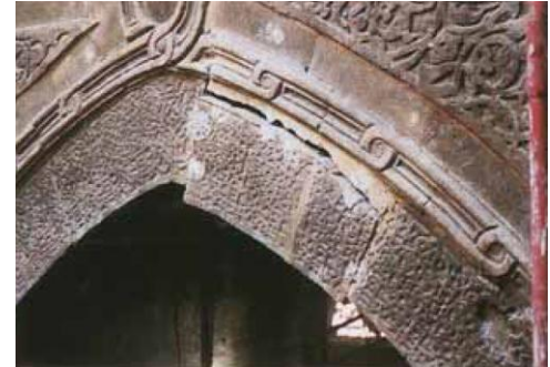
Seismic damage to decorative arches
