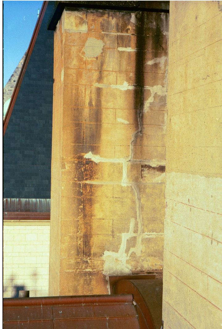
Failure due to hard mortar repointing
