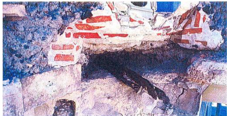
Once the cornice had been partially disassembled, the materials and techniques used in its construction could be easily identified. Note the linker concrete, or "bondcrete," between the terra-cotta blocks and the brick backup material and the cyclic deterioration of the steel supports. CSI recommended that all new rebarwork be type 316 stainless steel, a non-corroding type, which is essential in this chloride-rich maritime environment.
