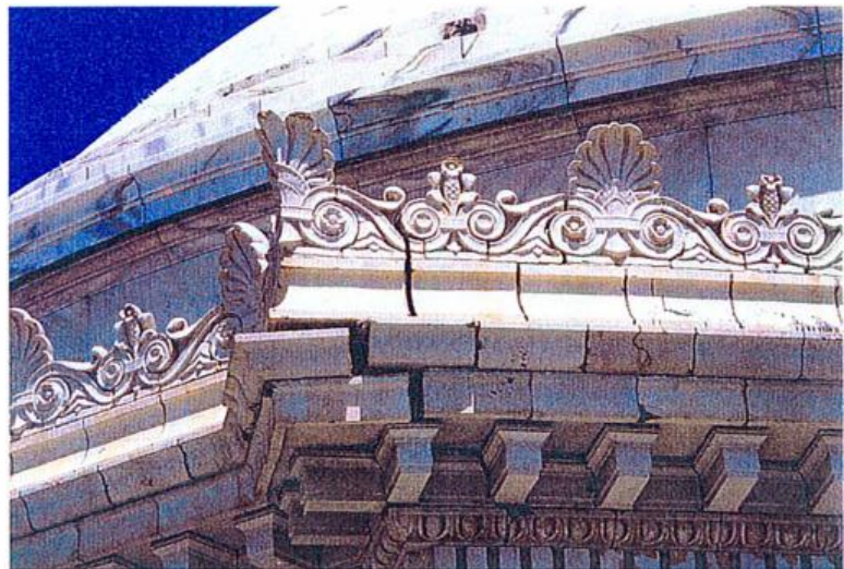
The poor condition of the terra-cotta cornice is evident in this view. The separation of the terra-cotta units is due to not only the failure of the anchoring system, but also the expansion of the corroded material.
